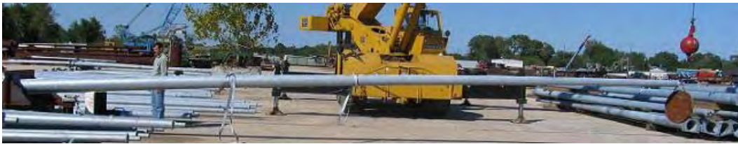
Figure 6 Entire Loaded and Fixed Mast Arm UIT Setup
