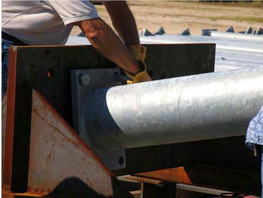
Figure 2 Mast Arm Being Connected to Fixed Testing Stand
