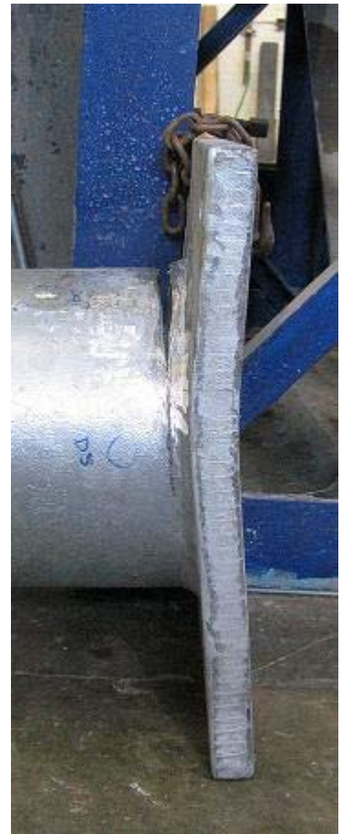
Figure 5: Side View of Mast Arm TXuDLGP After Cracking
