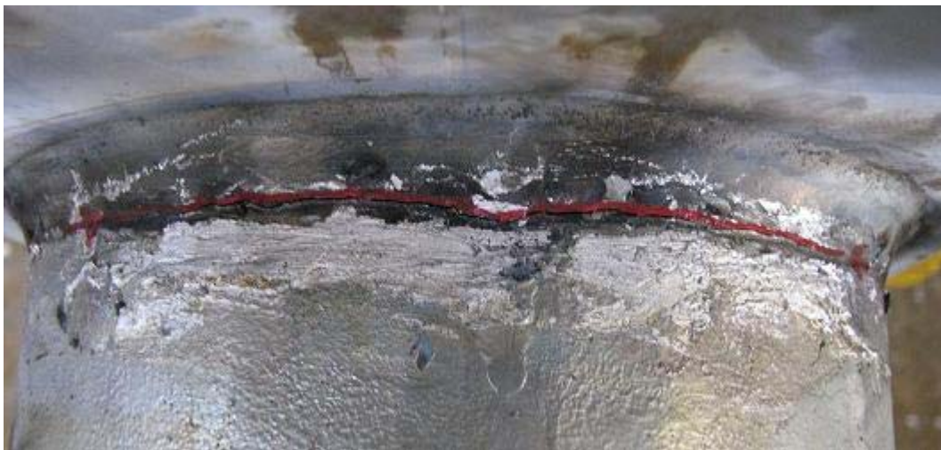
Figure 9: Highlighted Fatigue Crack at Weld Toe
