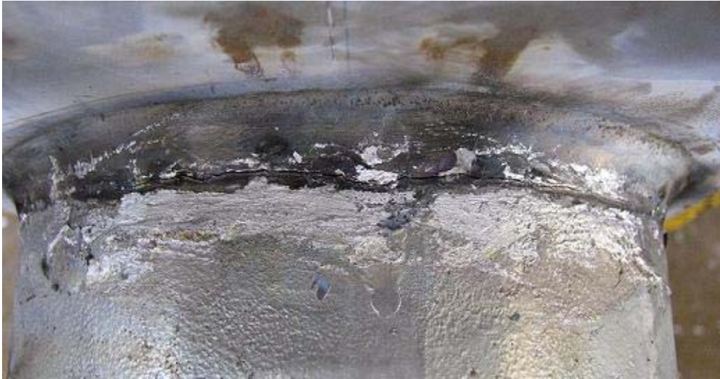
Figure 8: Mast Arm After 117,461 Cycles and After Removal of All the Repair Coating
