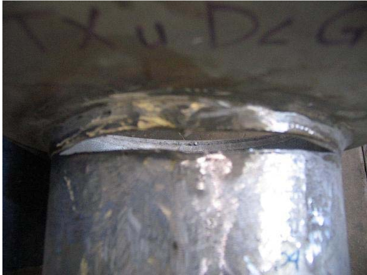
Figure 4: Top View of Crack at Weld Toe of TXuDLGP
