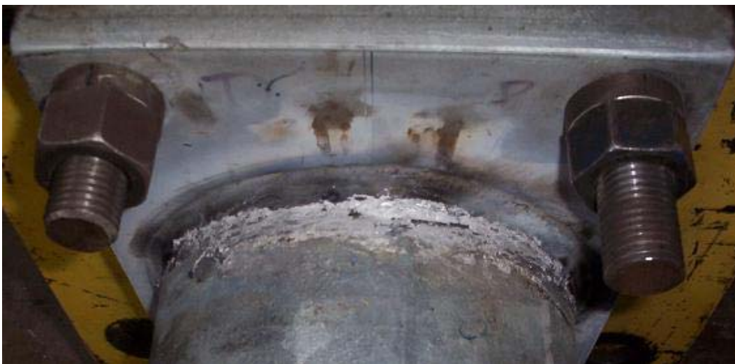
Figure 7: Mast Arm TXuCLGP After 109,411 Cycles
