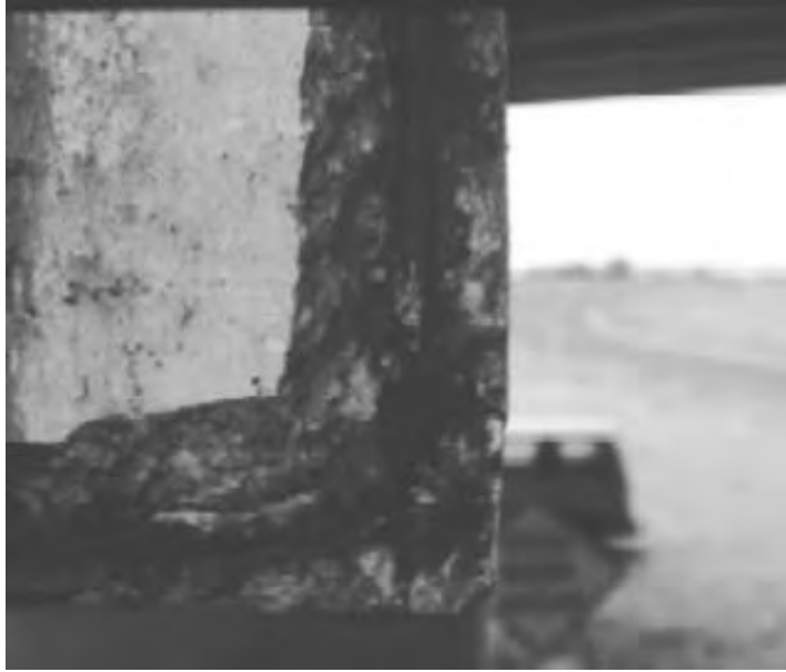
Figure 5.11 Closeup of area with severe concrete spalling
