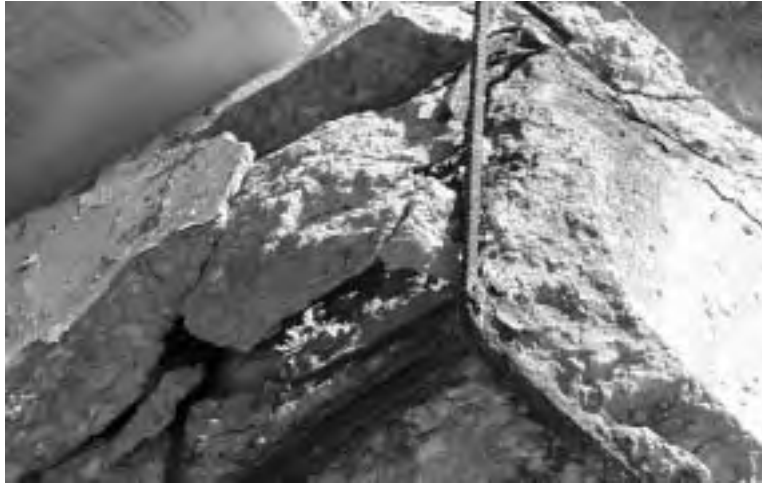
Figure 5.2 Closeup of corrosion damage on Structure #8
