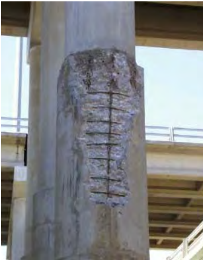
Figure 5.12 Concrete spalling on a bridge support column
