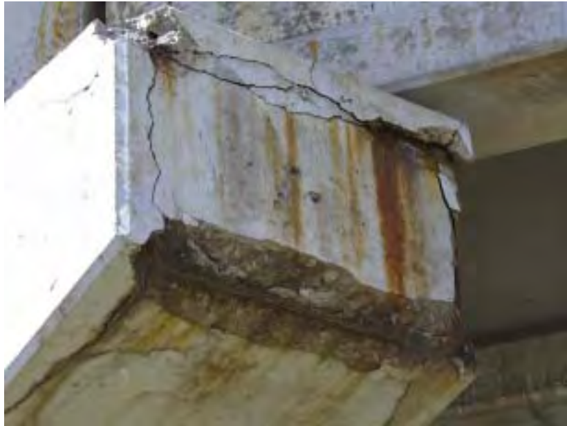
Figure 5.1 Endcap damage to Structure #5
