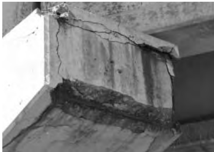
Figure 1.2 Damage at downstream endcap
