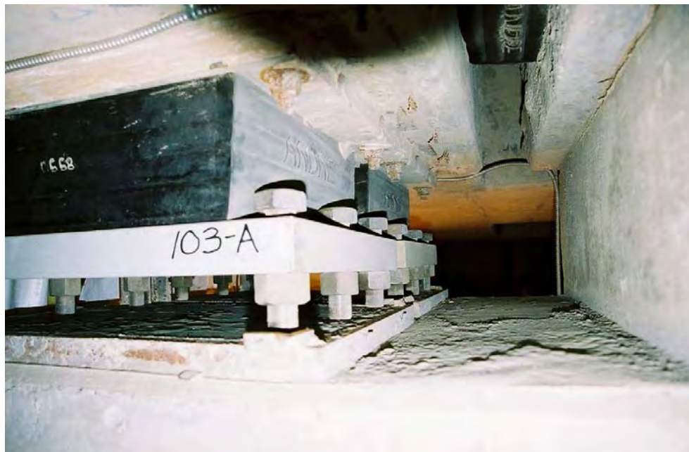
Figure 1. Rubber bearing, which absorbs vibration from nearby tunnels
