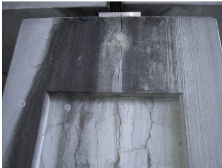
Figure 1.2 DEF in a column in San Antonio, TX
