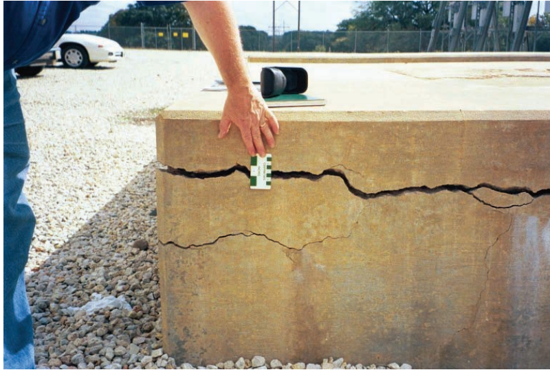
Figure 1.3 ASR in a transmission tower foundation in La Grange, TX
