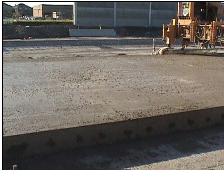
Figure 4-14: Concrete debris caused by tining over an already set concrete surface
