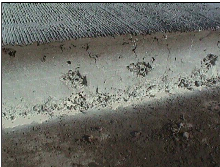
Figure 4-16: Cracking in the fresh concrete on the edge of the section placed on 8/7/00
