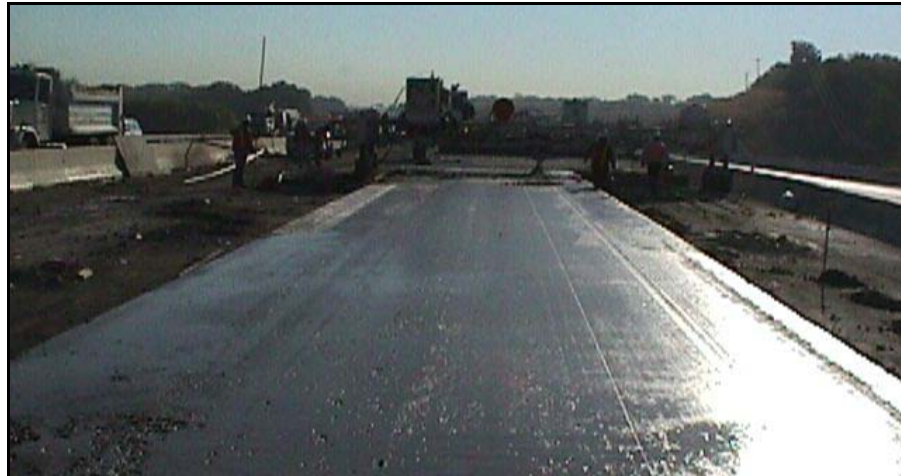
Figure 3-18: The accumulation of bleed water on the surface of a newly paved section
