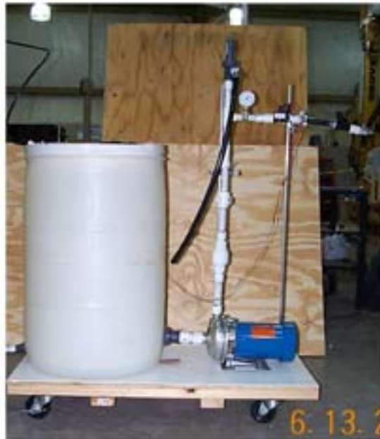
Figure 5. Pump, reservoir, piping.
